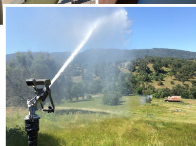
Irrigation Pump Station
