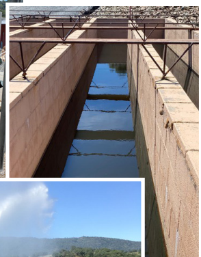
Chlorine Contact Basin
